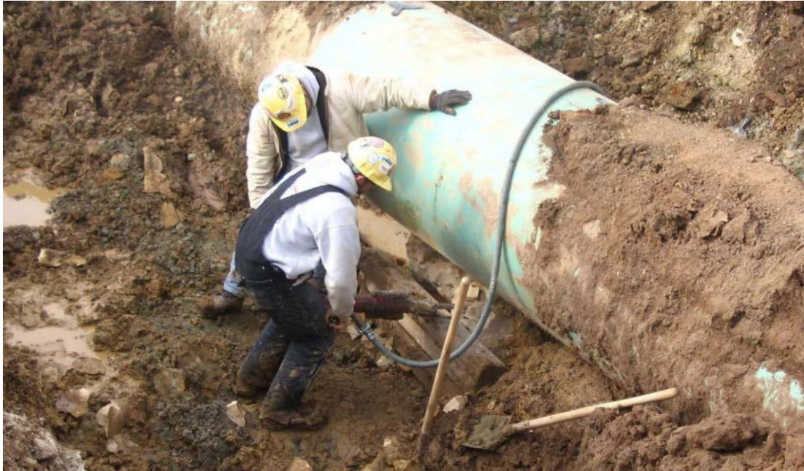
Figure 14: Repair of large diameter pipeline, removal of rock (Source: U.S DOT PHMSA)
