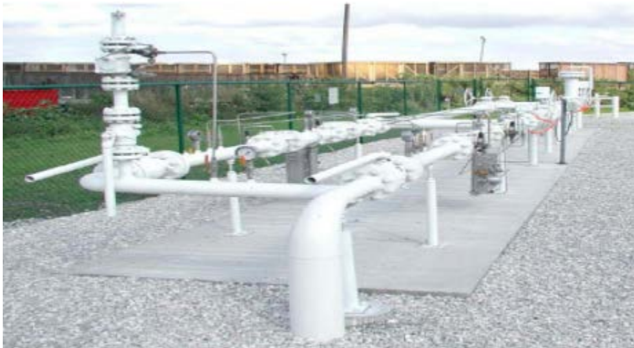
Figure 10: City gate gas measurement and regulating station
