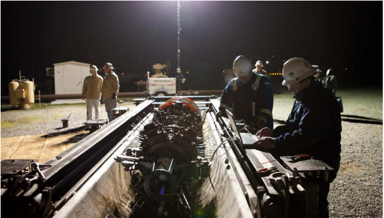
Figure 12: Large diameter inline tool (Source: Courtesy of Sempra Energy)
