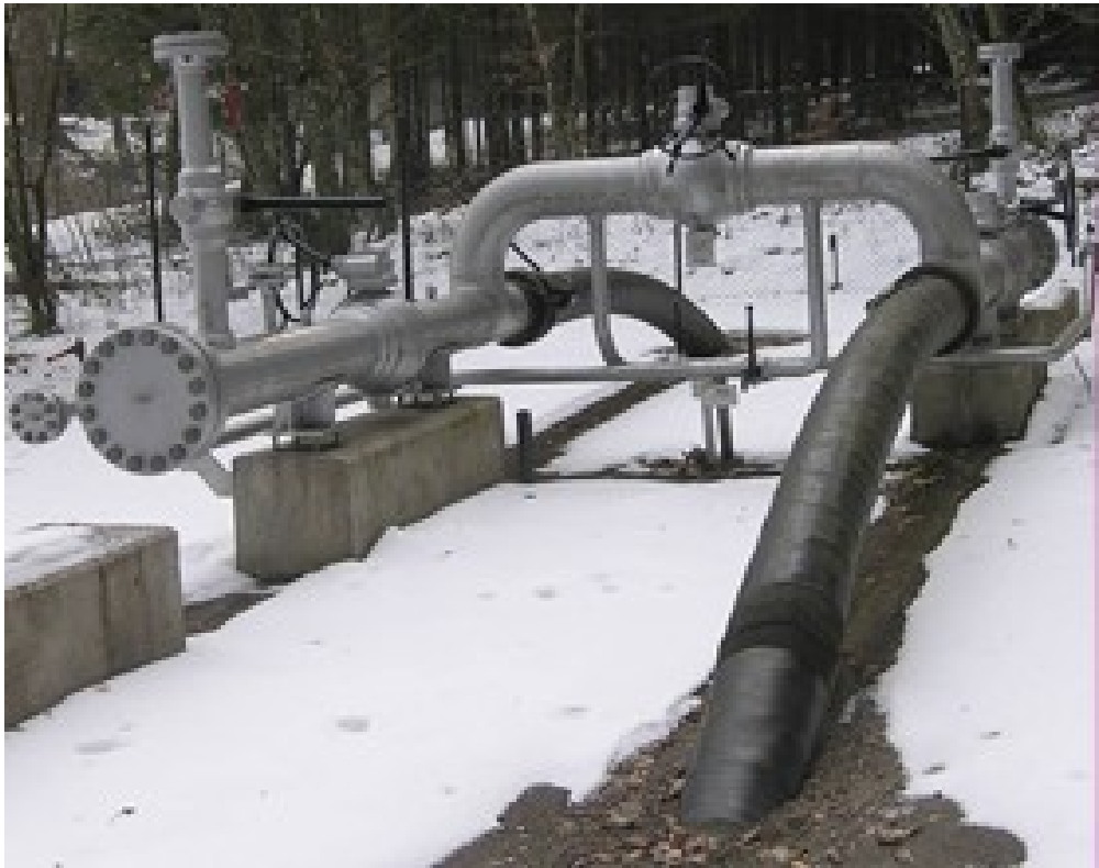
Figure 11: Inline tool launcher/receiver
