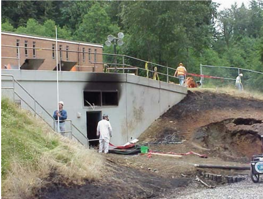
Figure 17: Water Treatment Plant Damage, Bellingham, WA (Source: Used with permission from the Whatcom County Photo Archives )
