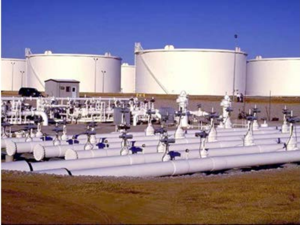
Figure 8c: Hazardous liquid tank farm (Source: U.S DOT PHMSA, Introduction to Pipelines )
