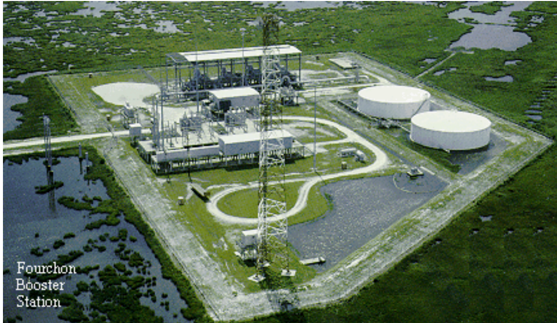
Figure 8a: Hazardous liquid pumping station (Source: Louisiana Department of Transportation and Development, http://www.dotd.la.gov/programs_grants/loop/ )
