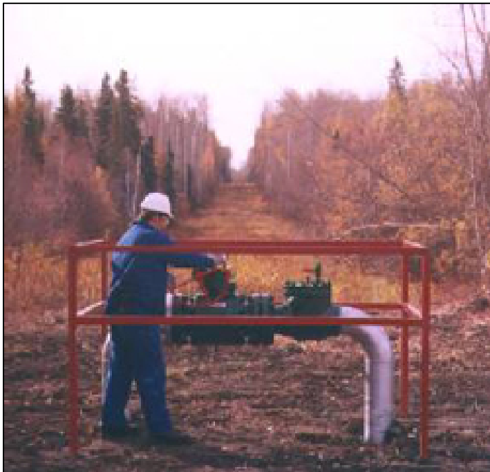
Figure 9: Aboveground Valve on Natural Gas Pipeline
